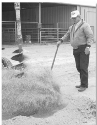
Kasper overseeing digging of post holes during an expansion phase of the Live Oak barn.
